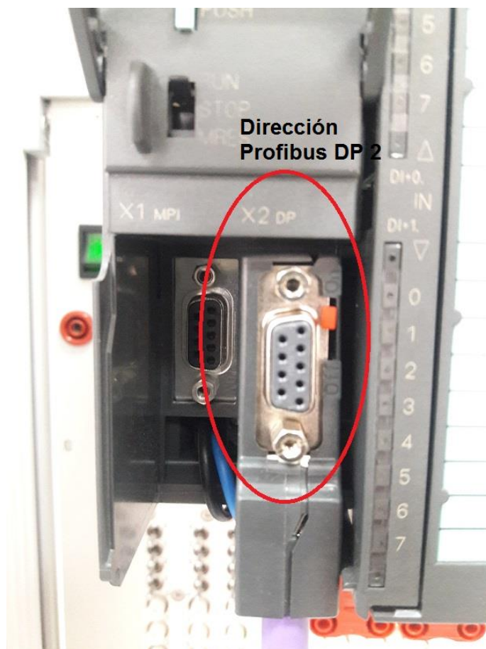
Figura 30: Conector X2 DP del PLC
