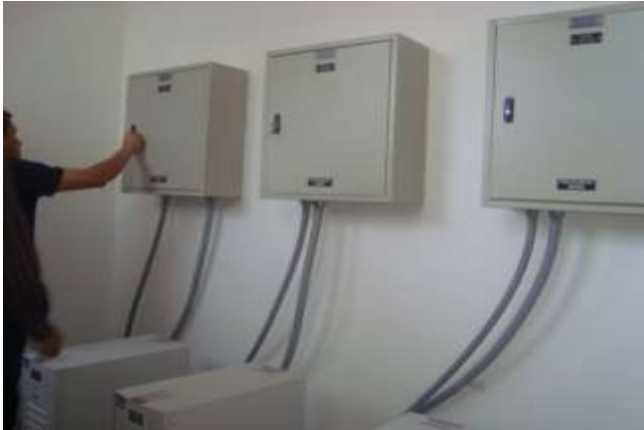
Figura 40. Paneles de control UPS UMI
